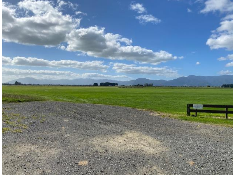
Photo 3: Gap in Fencing at Entrance to Aerodrome
